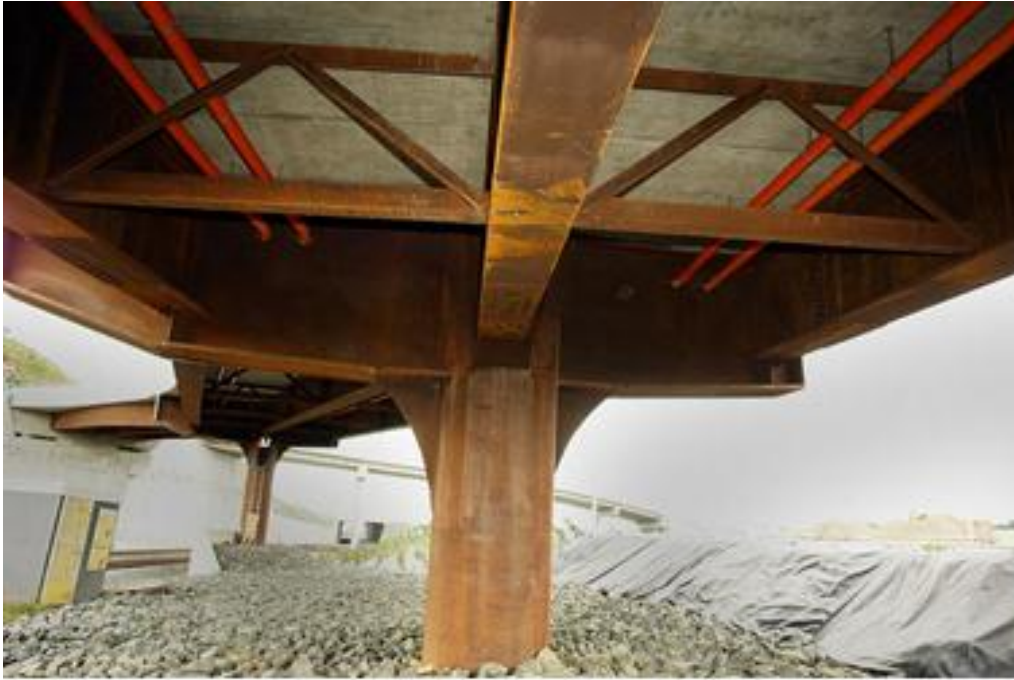
Figure 1: New Zealand's first weathering steel bridge (State Highway 1 Mercer to Longswamp Off-ramp, opened in 2006)
