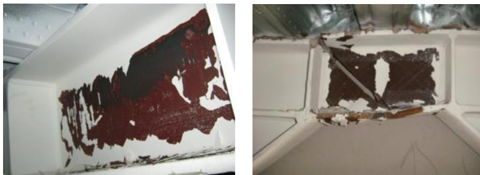
Figure 1. (Left) Paint flaking of the most heavily strained EBF link in Club Tower, Christchurch, (Right) Fractured link at level six of Pacific Tower, Christchurch
