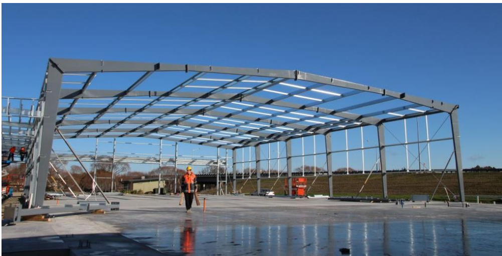
Figure 2. A new DGL build North of Christchurch for PlaceMakers using the NTBB, 30m clear span.
