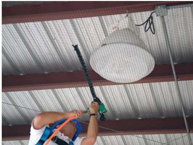
Figure 5. An example of the installation methods for bird proofing. Access is being added to roof space in a building using bird netting and hot rolled section frame.
