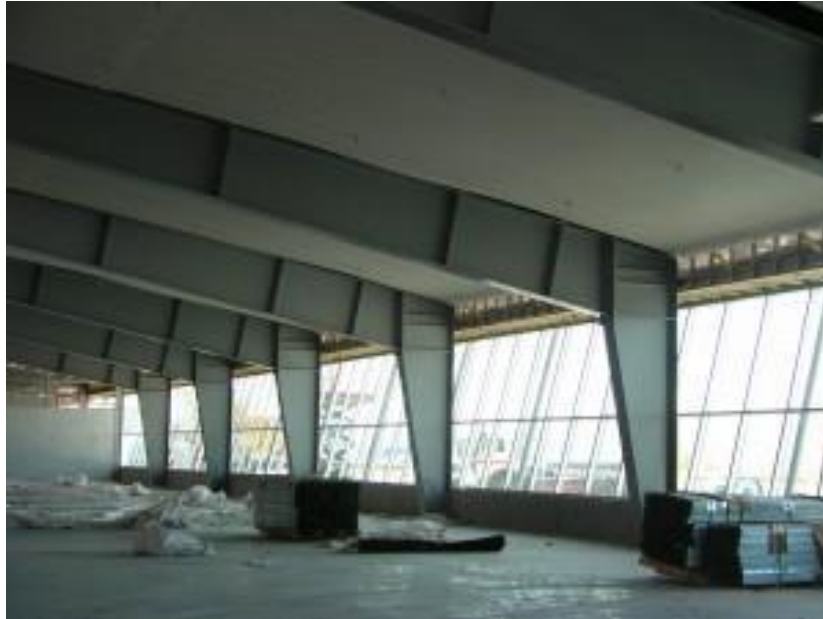
Figure 1. Custom welded beams produced by Steltech. NZ Post sorting room Highbrook Business Park, 60m clear span
