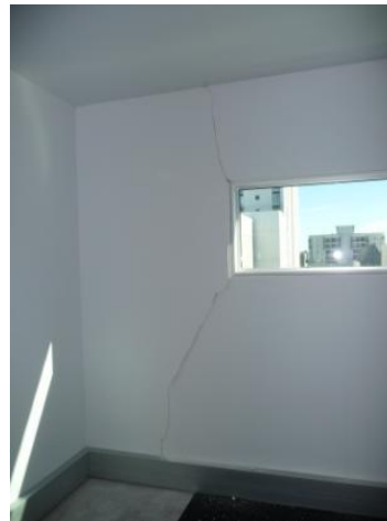
(b) Cracking to internal linings of a window-box [C Clifton]
