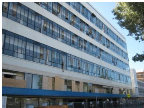
(a) Structural and claddings damage [J Ingham]
