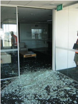
Figure 4 Dislodged glass door due to vertical acceleration [C Clifton]
