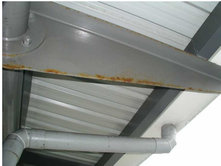
Figure 3: Sharp Edges Accelerated Corrosion
