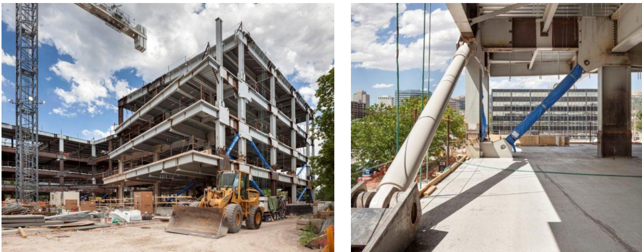
Figure 1 – New construction of the Salt Lake City Public Safety Building, a post-disaster performance level steel moment building frame using fluid viscous dampers (Holmes Culley, San Francisco).
